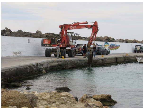
Figure 8.1. Drilling to create more berthing space within the modern harbour of Hierapytna poses a threat to the remaining fragments of the Roman imperial harbour and has destroyed the natural rock formation that was part of the entrance into the ancient harbour (photo by Michael J. Curtis).*
